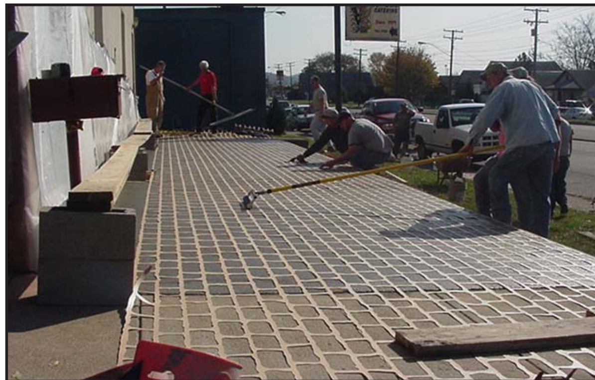
FINISHING UP A COURSE in stenciling in Charleston are members of Cement Masons Local 887.
